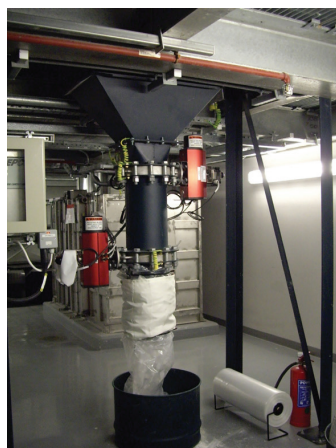
BIBO for Dust Discharge
